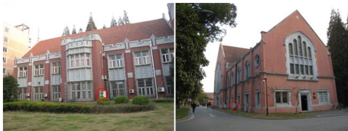
Fig. 1. Air-conditionings units making great damages to HB facades.
