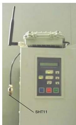
Fig. 7. The temperature and humidity sensor node placed in spot.
