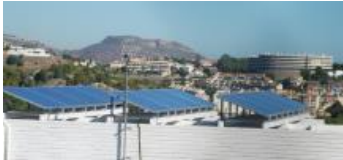
Fig. 1. View of the photovoltaic installation.
