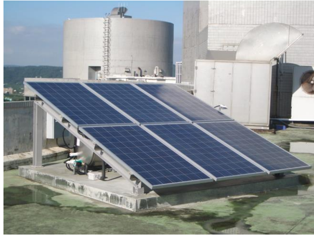
Fig. 1. 1.44kW/500L photovoltaic thermal hybrid system.
