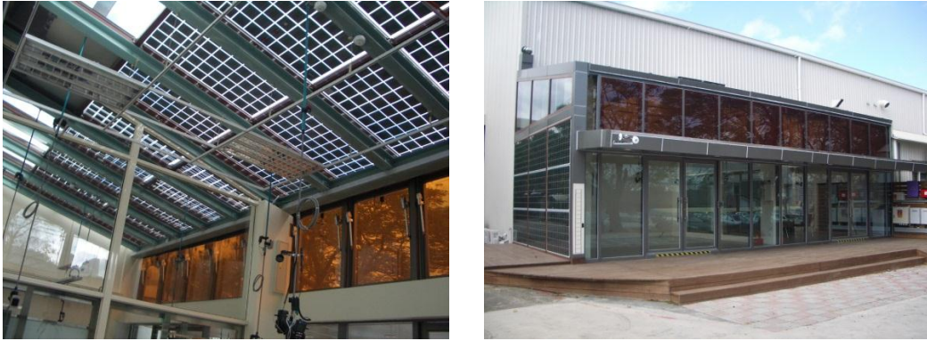
Fig.2. Semi-transparent c-Si PV module in tiled roof has 4.2kW installation capacities.
