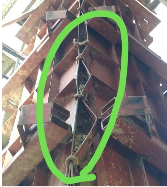
Fig. 2. Deformation at the edge of the column formwork.
